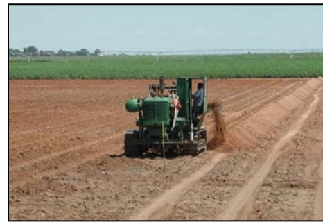
Figure 3. Opening ditches with a Cleveland trencher for water supply and flush manifold connections to SDI laterals.
