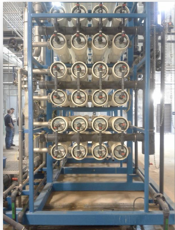
Figure 5-7: Microfiltration and reverse osmosis treatment units at Colorado River Municipal Water District Raw Water Production Facility, Big Spring, Texas
