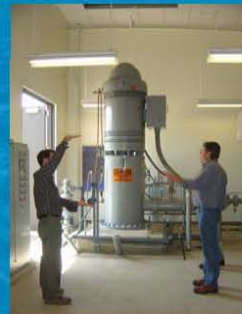
Calleguas MWD, Thousand Oaks, California ASR Well
