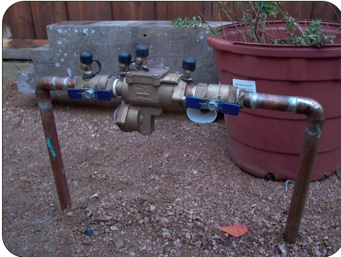
Backflow prevention device, McMahan residence, Dallas, Texas.
