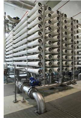
Reverse osmosis system
